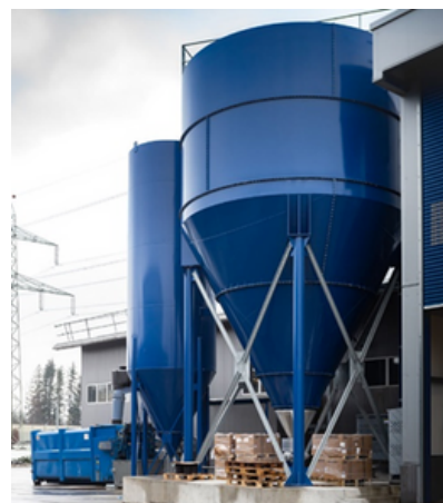
Clear water stocking tank
